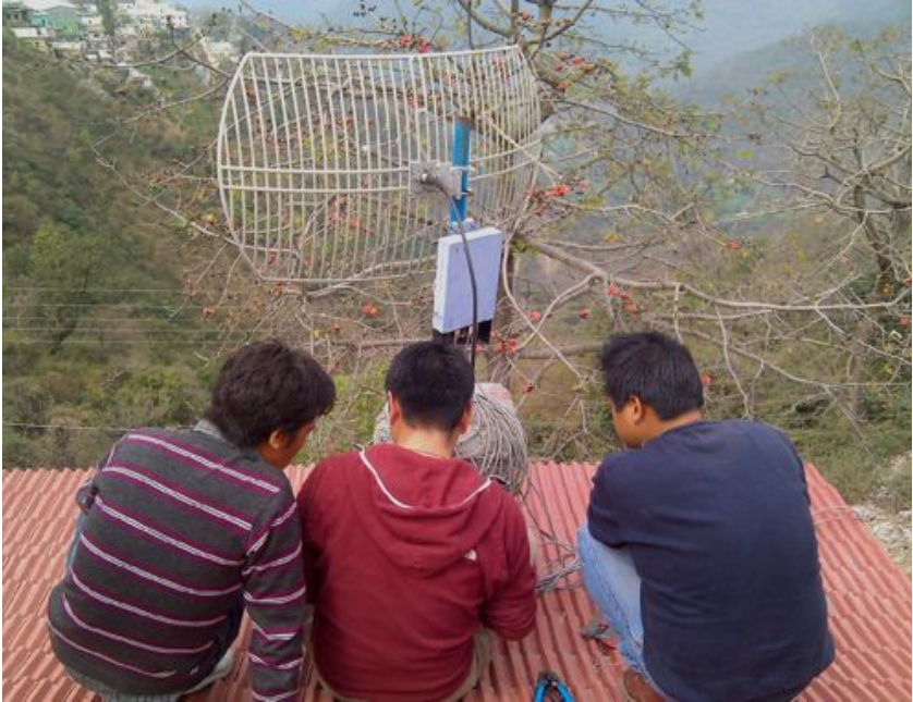
Figure CSD 6: Relay troubleshooting, Kumaon Network
