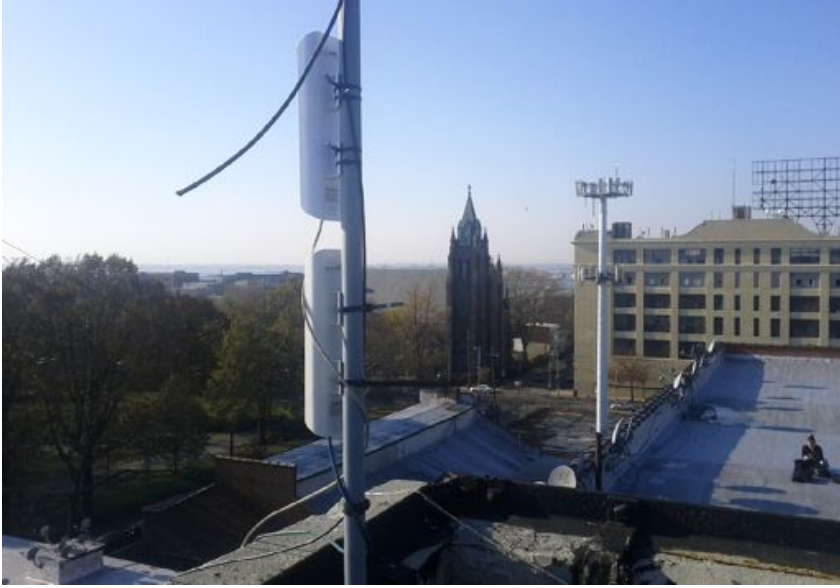
Figure CsOTI 14: Rooftop node installed after Superstorm Sandy.
