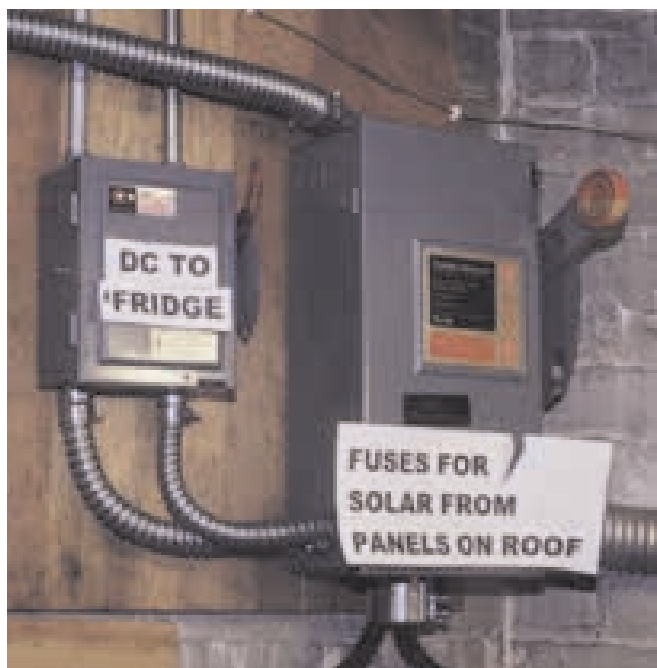
Left: DC distribution. Right: PV disconnect.
